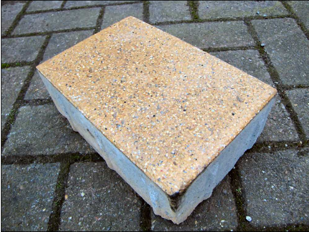
Figure 34 - Block showing tyre marks remaining on arris after cleaning
