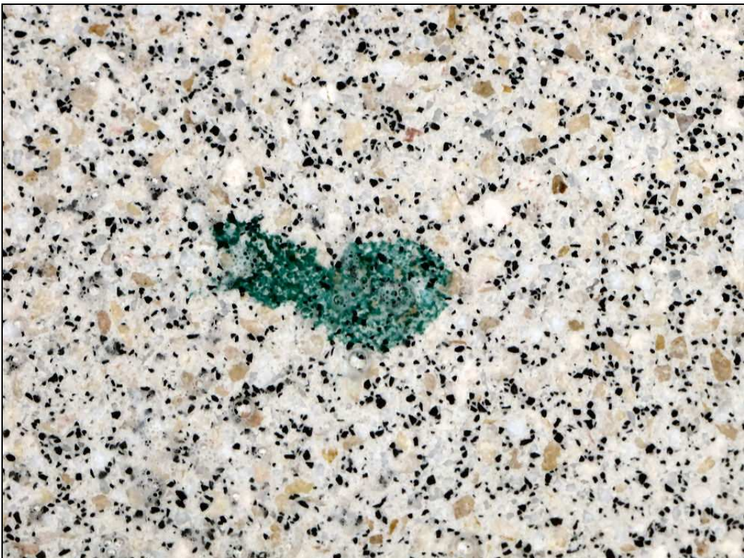
Figure 18 - Permanent staining caused by timber preservative
