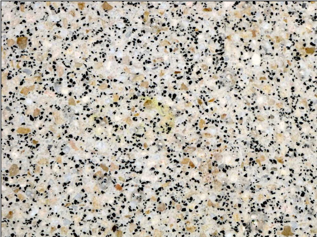
Figure 17 - Faint staining from mustard was cleaned by scrubbing
